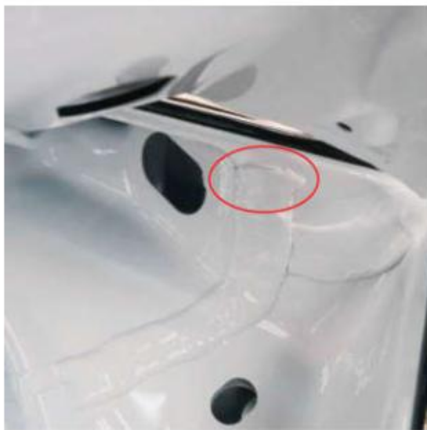
图1 PVC胶开裂缺陷的目视表现 Fig.1 Appearance of PVC glue crack defect
